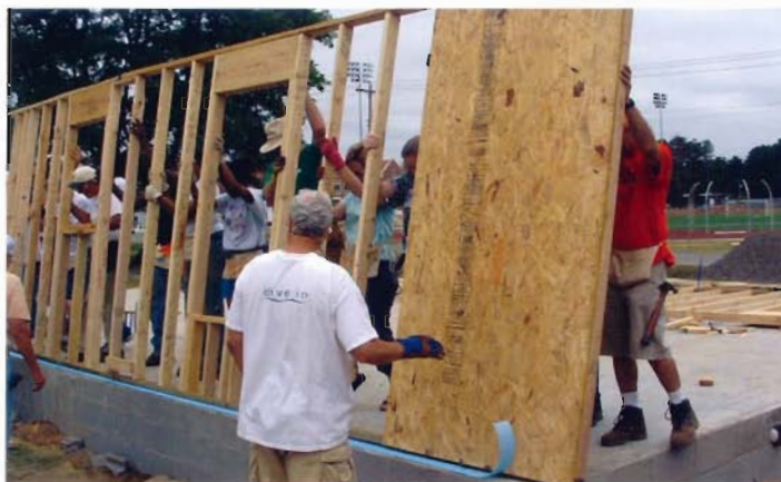
Volunteers position a wall for Habitat home. Six local churches have volunteered to help build a home in Conway through Habitat for Humanity.
